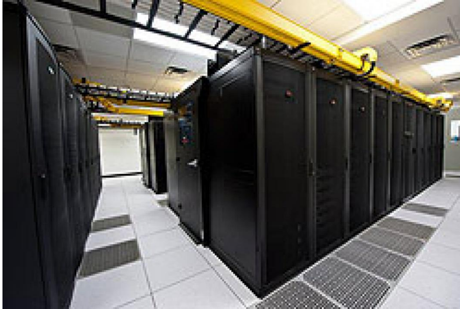
Figure 7: Data Center Racks (Source: DOE)
